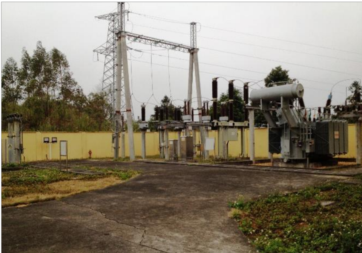
Figure 18.6 GC mine substation
