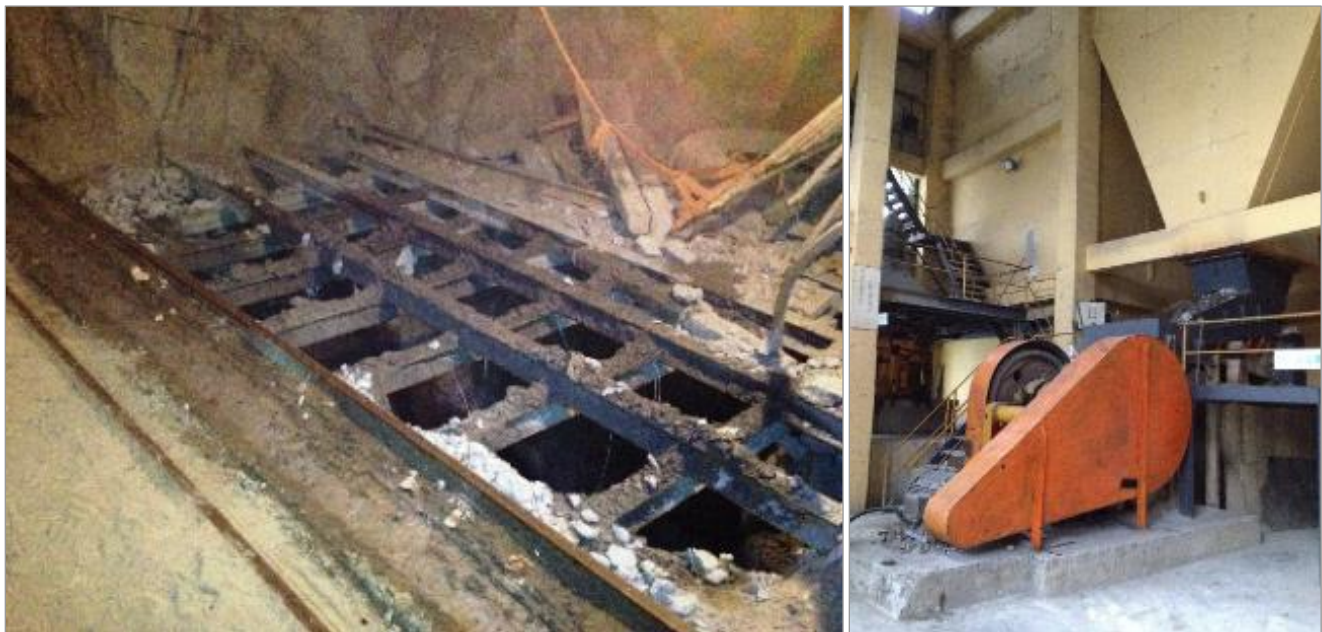
Figure 17.3 Surface grizzly feed to ROM ore bin
