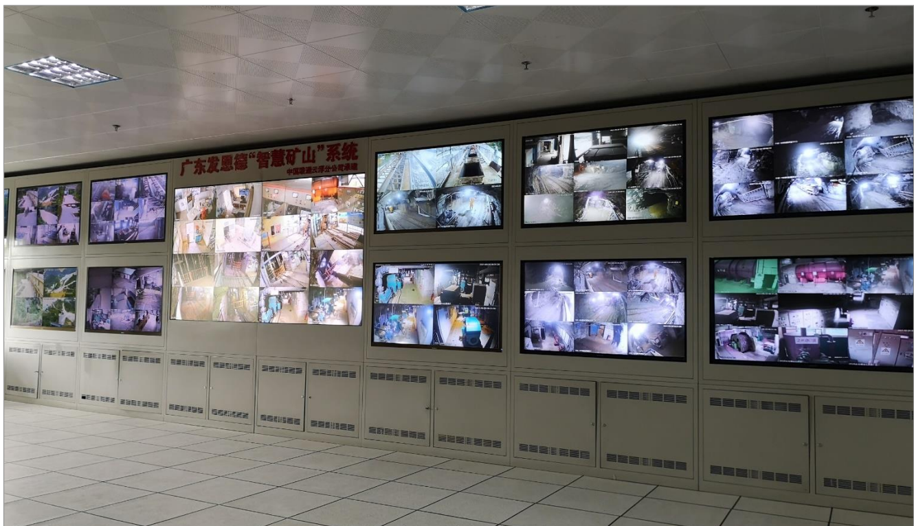
Figure 17.8 Control room screens
