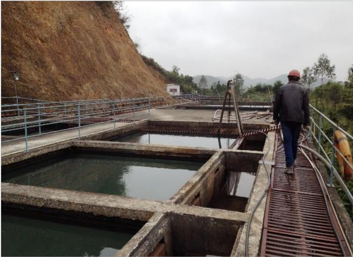
Figure 18.7 GC water treatment facility
