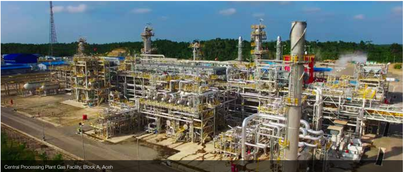
Central Processing Plant Gas Facility, Block A, Aceh
