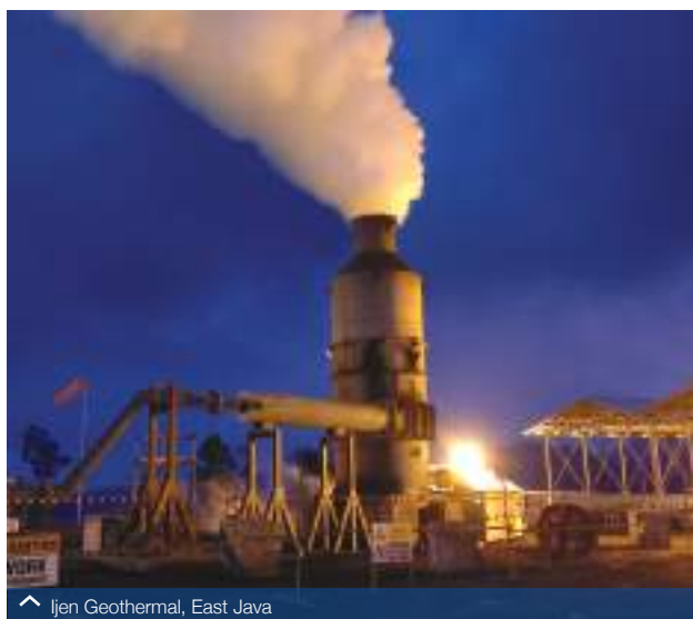
^ Ijen Geothermal, East Java
