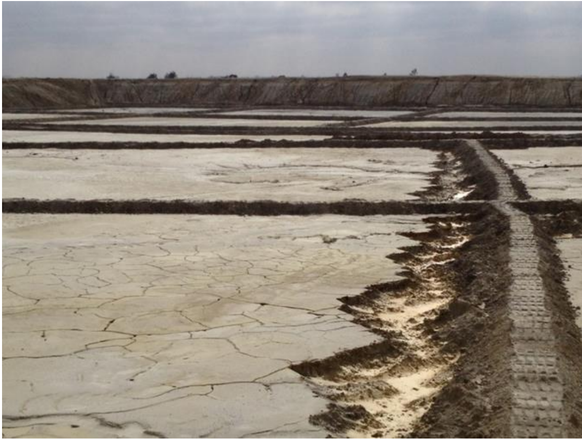
Figure 6.8: A Paddocked Facility, Illustrating How the First Cut's Outer Walls Are Left Intact to Contain Rain/Stormwater Inside The Facility
