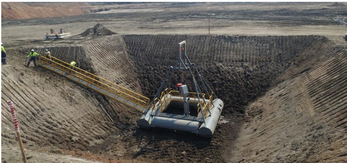
Figure 6.2: Typical Satellite Barge Installation
