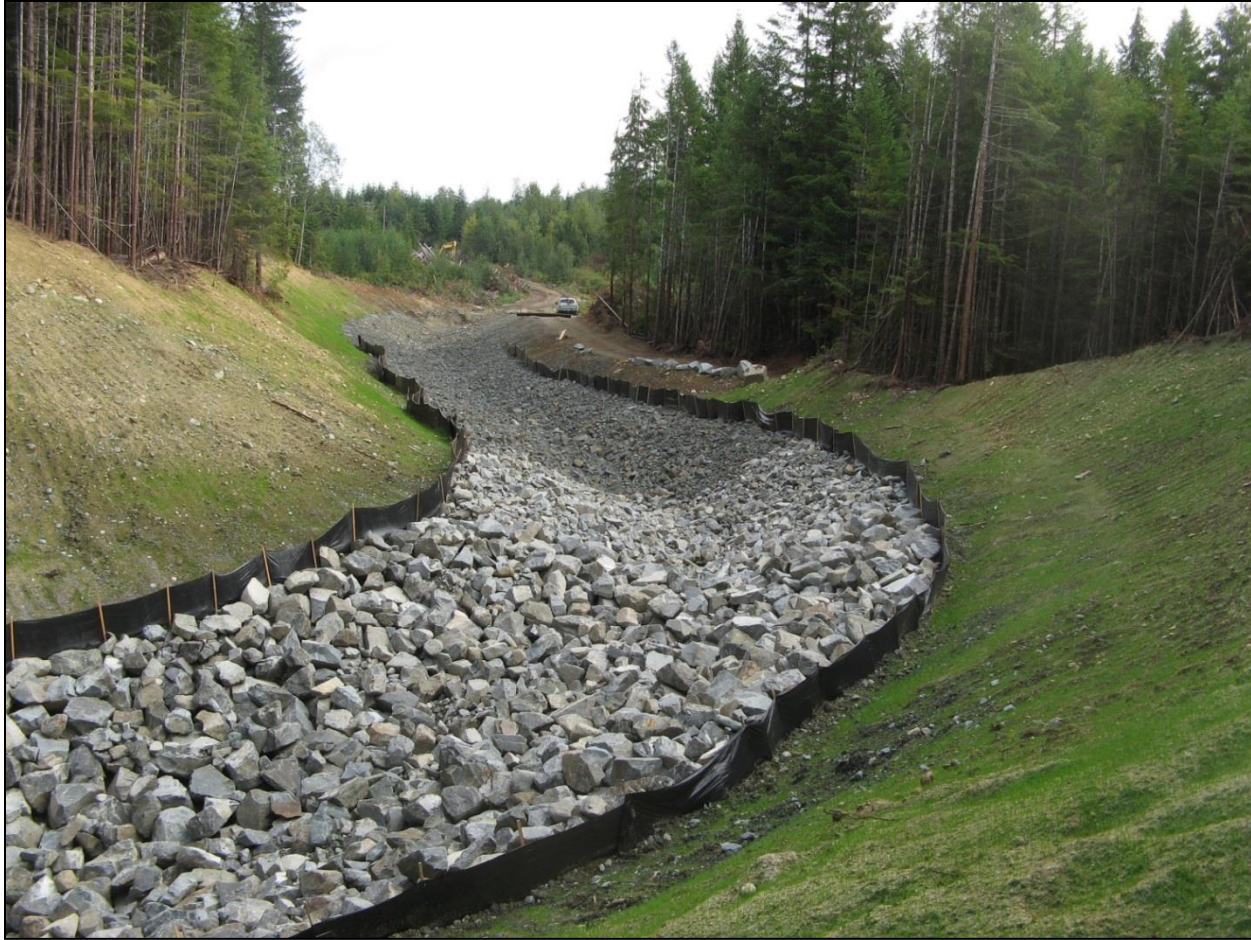
Figure 20: 3 South Pit Outlet Channel completed but inactive, displays the revegetation of the sloped walls, fall 2016. No scotch broom infestations.
