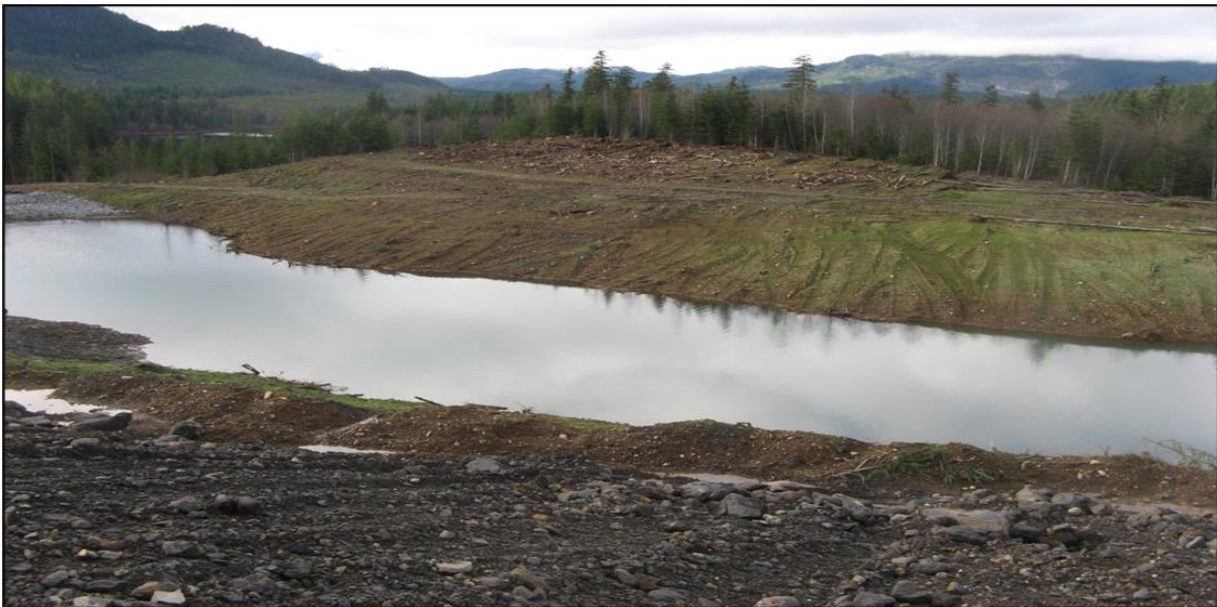
Figure 15: 3-South Pit Pond PAG-CCR Facility following the re-sloping and revegetation of the North Dump, fall 2016
