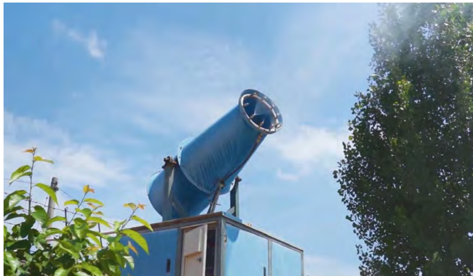
Fog cannon dust suppression system
