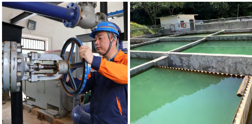
Inflow water pump room
