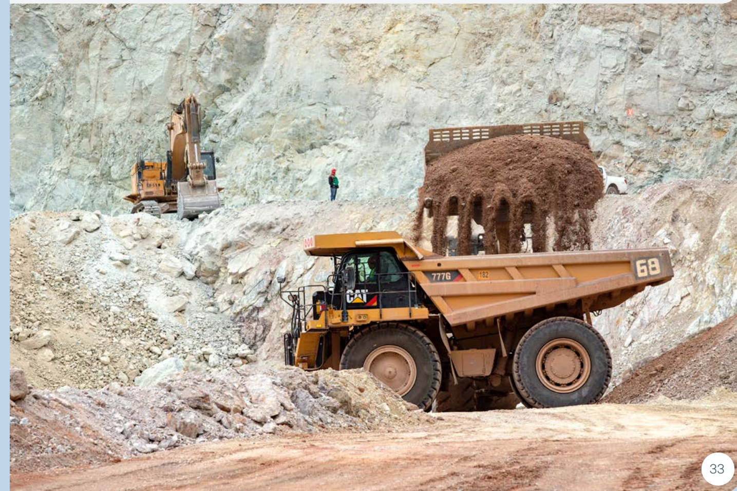
Haul truck loading in the open pit at the Mulatos mine, Mexico
