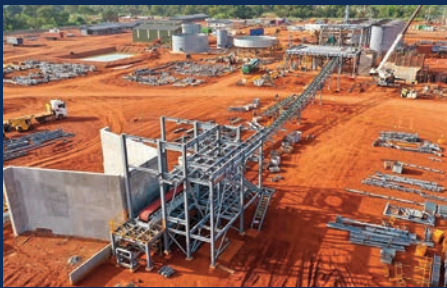
Assembly of the mill feed conveyor underway - October 2022 at Séguéla, Côte d'Ivoire
