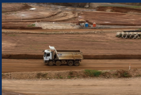
MVV has been ramping up at a strong pace since construction was completed in June 2021
