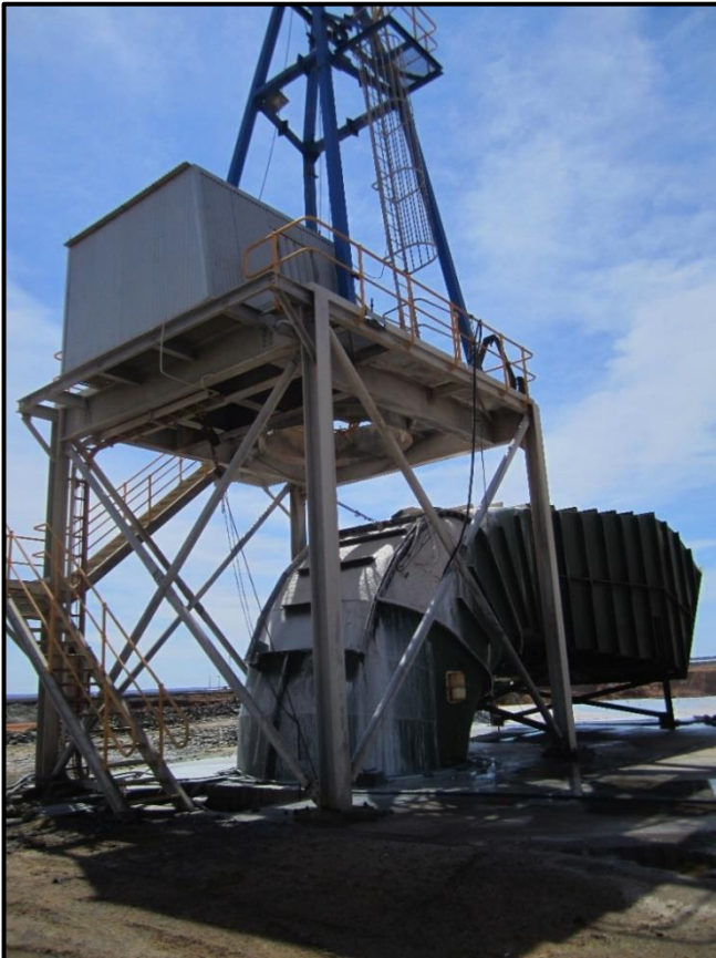
Figure 18.2: Beta Hunt return airway and emergency egress hoist
