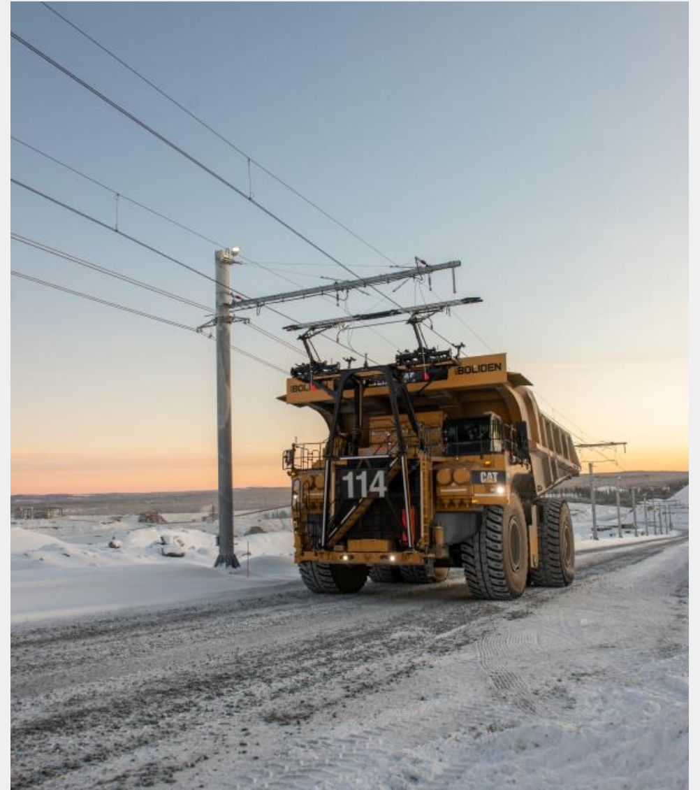
Electric trolley line, Aitik
