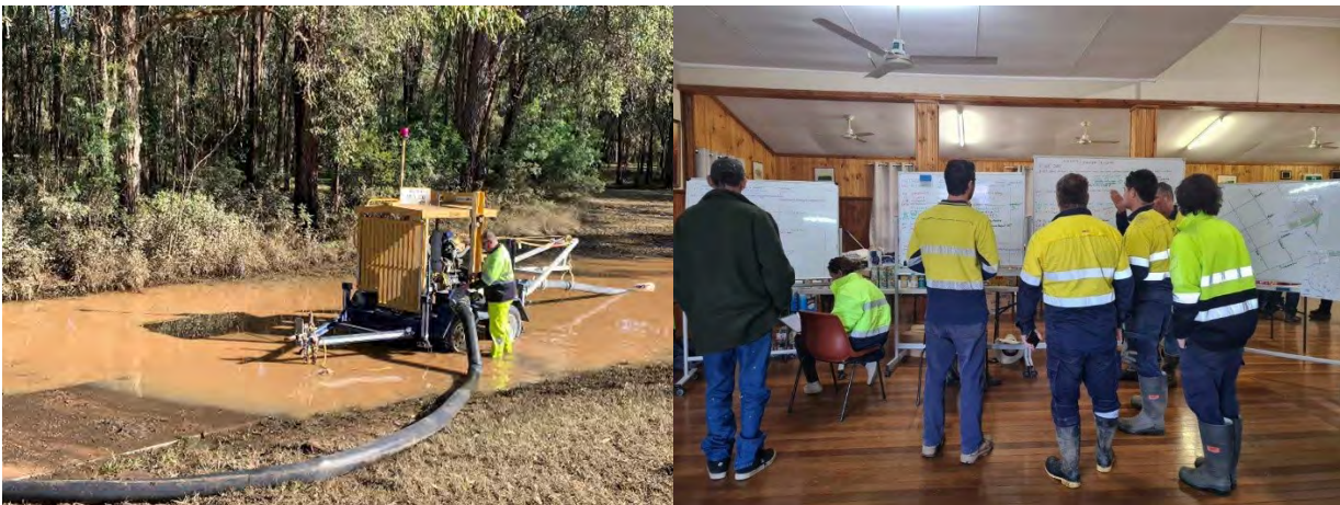
Photo 5 July 2022 Flood Event and Recovery
