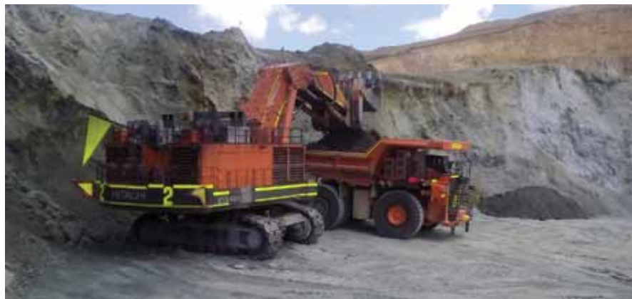
Hitachi equipment doing early works at Mina Justa. Photo courtesy of Zamine.
