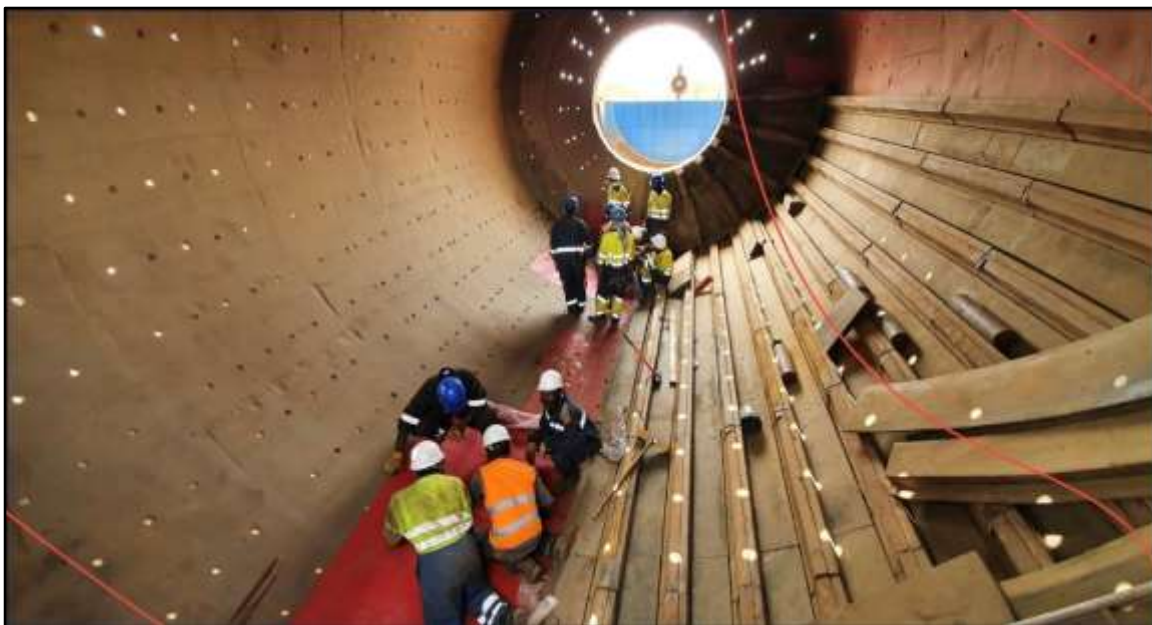
Plant refurbishment progressed well during the quarter including relining of the Ball Mill
