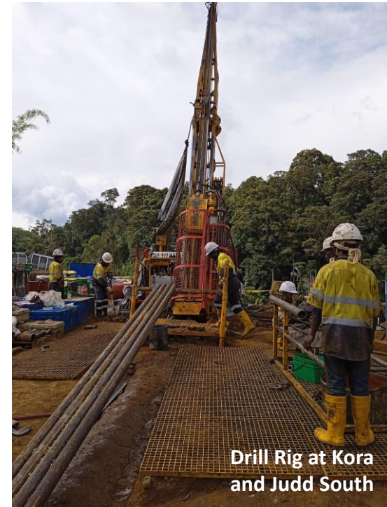
New Equipment Operating in Twin Incline
