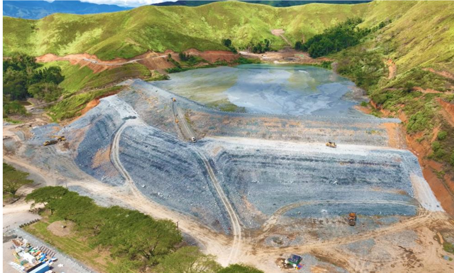
Recent Aerial of Yonki Dam tailings storage facility. Tailings dam lift 1C is underway and +60% complete.
