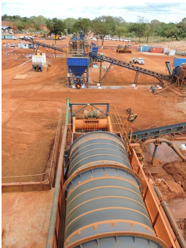
Figure 3-34: MRM: Wet scrubber screen
