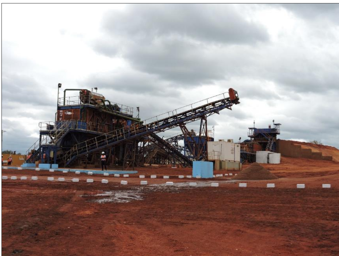
Figure 3-36: MRM: DMS plant and discard conveyor
