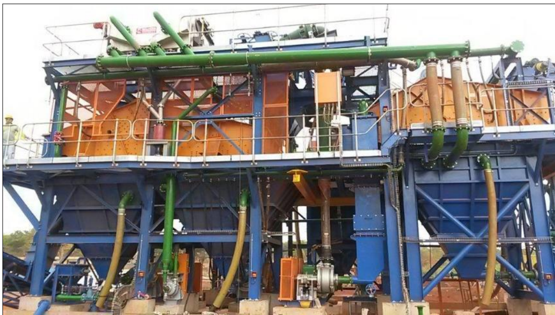
Figure 3-35: MRM: DMS plant showing feed screen, media pumping circuits, dense media cyclones and drain and rinse screen
