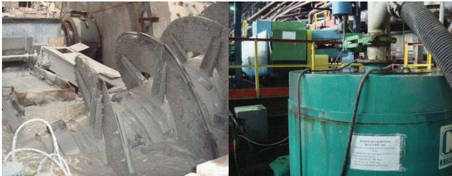
Photo 5.4: Jig on Mill Discharge (centre left) and New Knelson Concentrator
