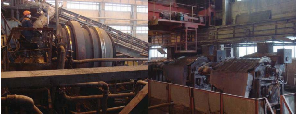
Photo 5.2: DMS Drum and Magnetic Roll Separators
