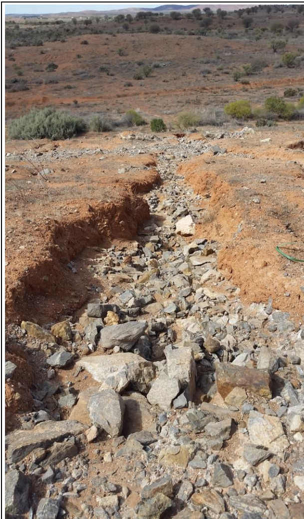
Plate 2 Erosion on the Batter of the Potosi WRE
