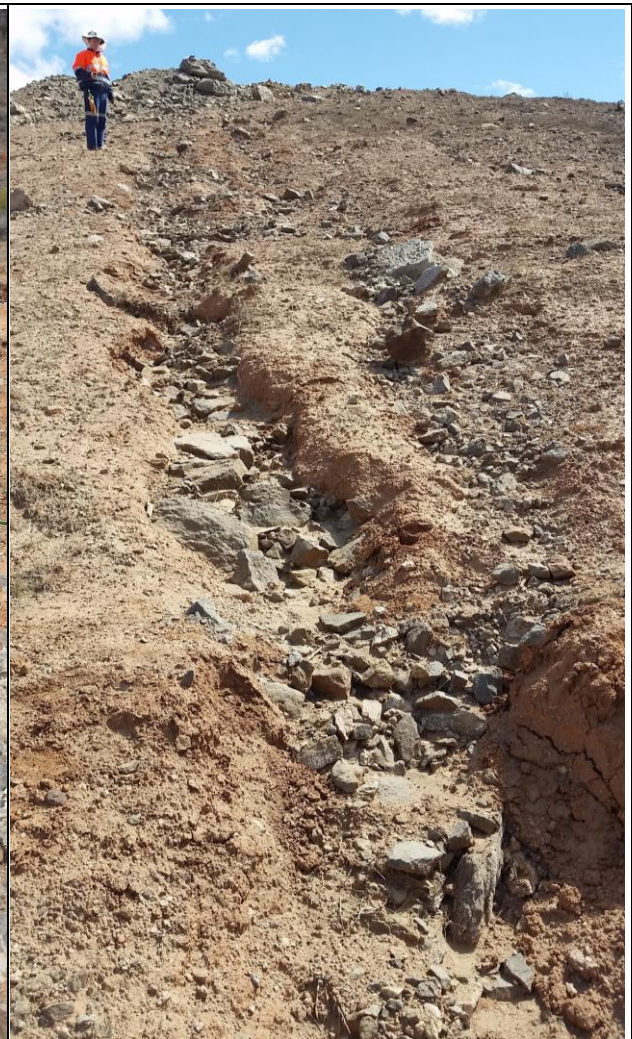
Plate 3 Erosion on the Batter of the Potosi WRE
