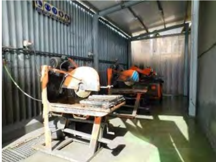
Figure 11-7: Core Sawing facility (Atalaya, 2022).
