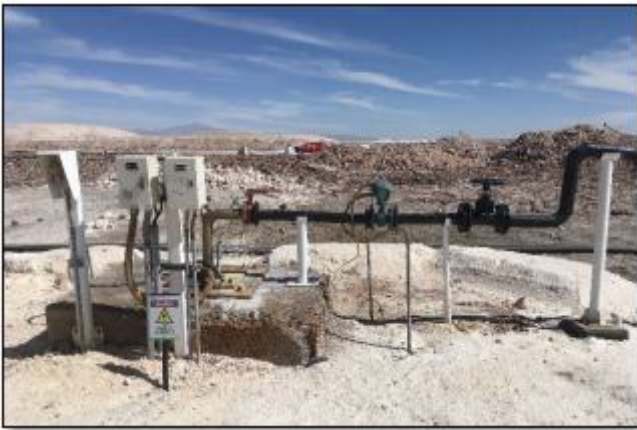
a) Brine production wells with surface equipment
