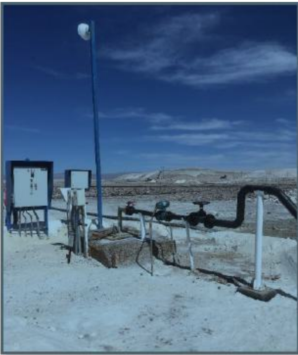
c) General view of a production brine well with an additional system for monitoring and control (telemetry)
