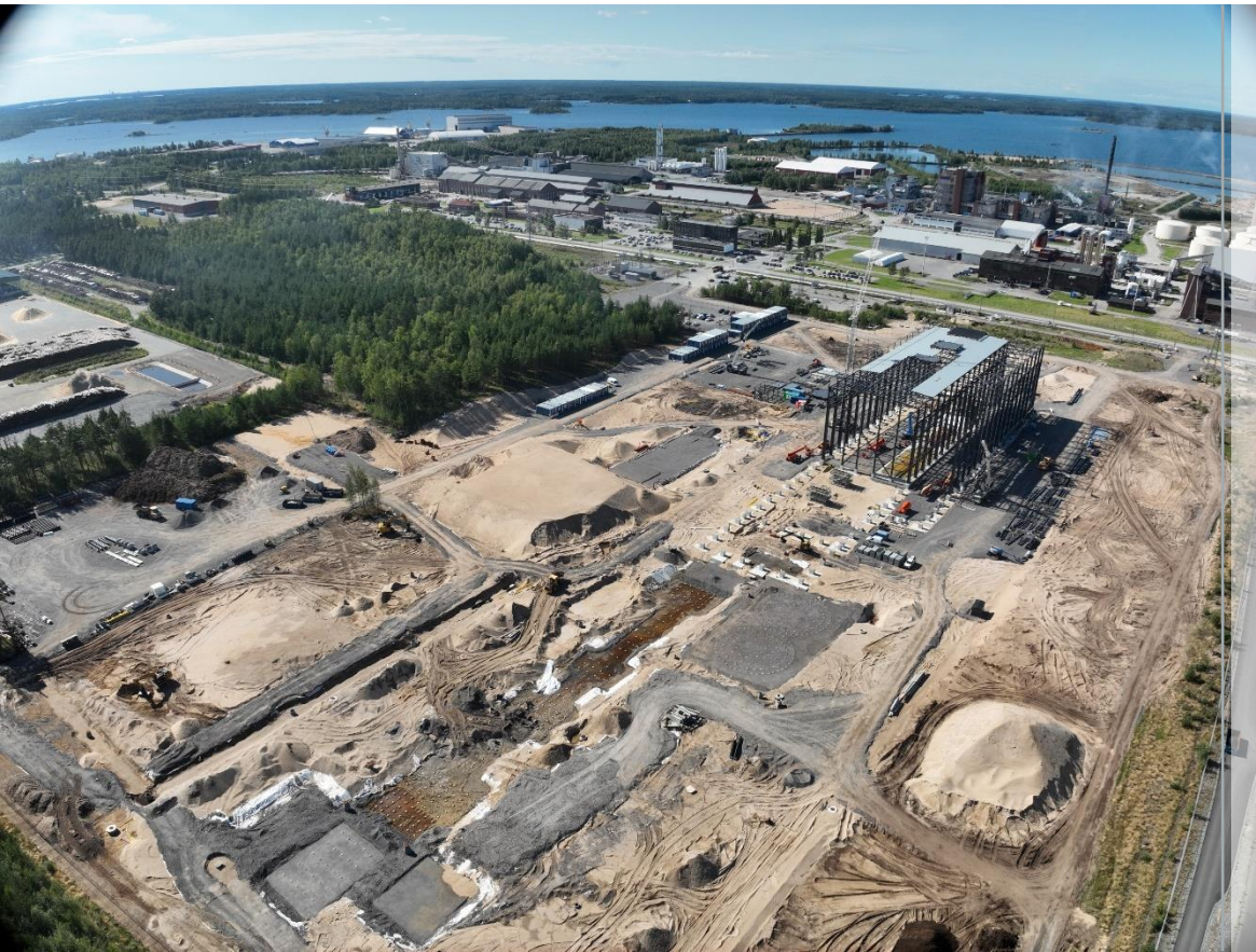
Aerial view of the construction at the Keliber lithium refinery August 2023 (credit: Tallqvist)
