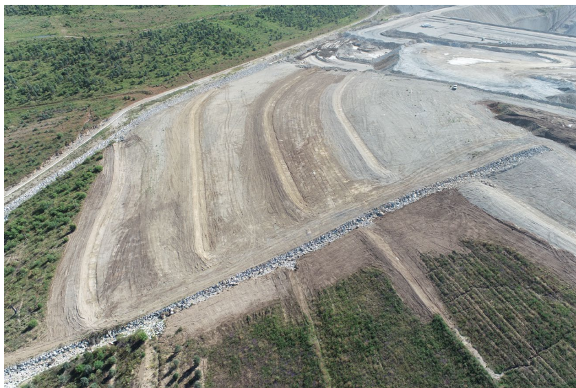
Figure 15 - Photo: Rock-lined Drop structure and completed contours on the Northern Rehabilitation area prior to topsoil placement - December 2022.
