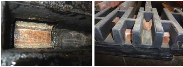
Figure 5—Old cell furniture (right), showing poor clearance between cap block and contact. On left is new cell furniture with robust contact clearance
