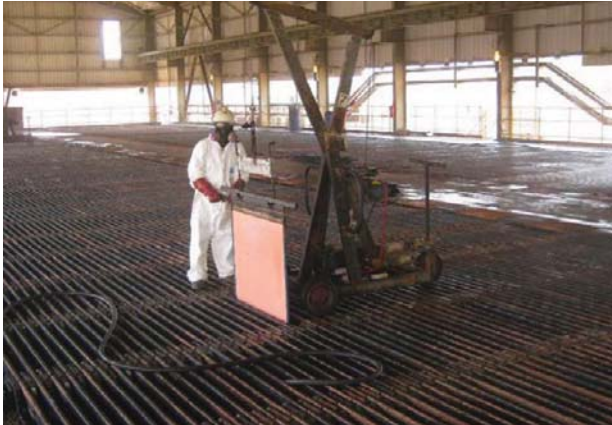
Figure 9—Single-pull cart used to correct short-circuits in tankhouse
