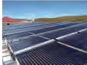
Renovated solar electric auxiliary heat boiler
