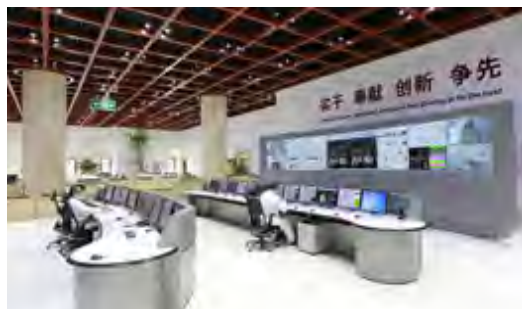
Beijing Gas-fired Power Plant's Centralized Control Center
