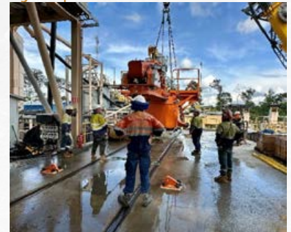
Figure 6 | Okvau Maintenance Personnel
