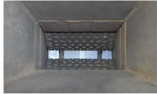
Feed Chute to Rolls
