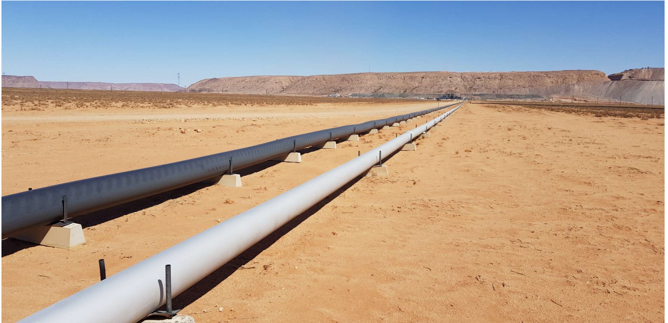
Figure 11: Example of overland pipes the concept planned for Kasiya (Source: Paterson & Cooke)
