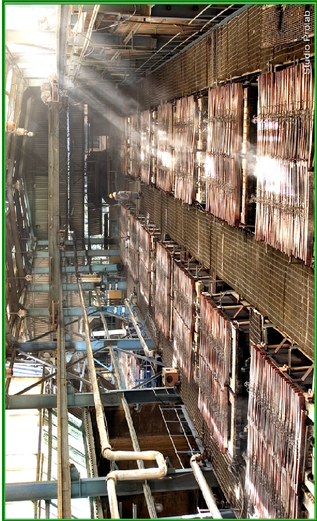
Arrangement of Electrolytic Cells at Electrolytic Manganese Dioxide Plant, MOIL Dongri-Buzurg Maharashtra
