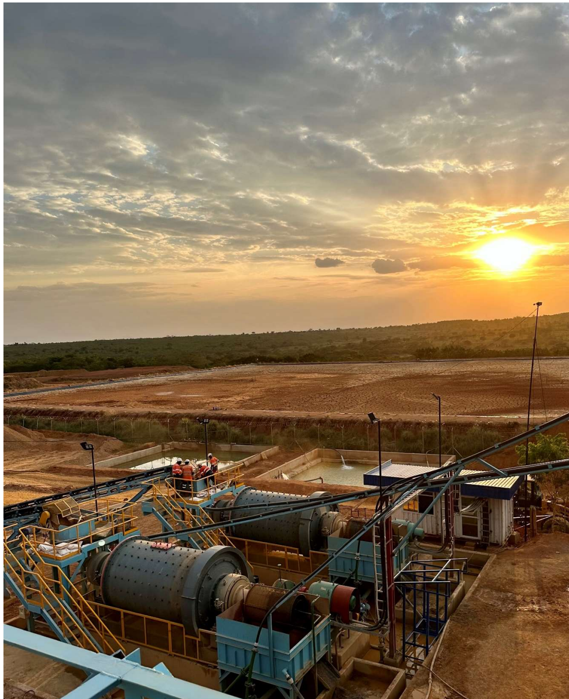
Figure 4: Buckeef Gold Expanded 1,000+ tpd Processing Plant, showing installation of two new 360 tpd ball mills (Q1 2023)
