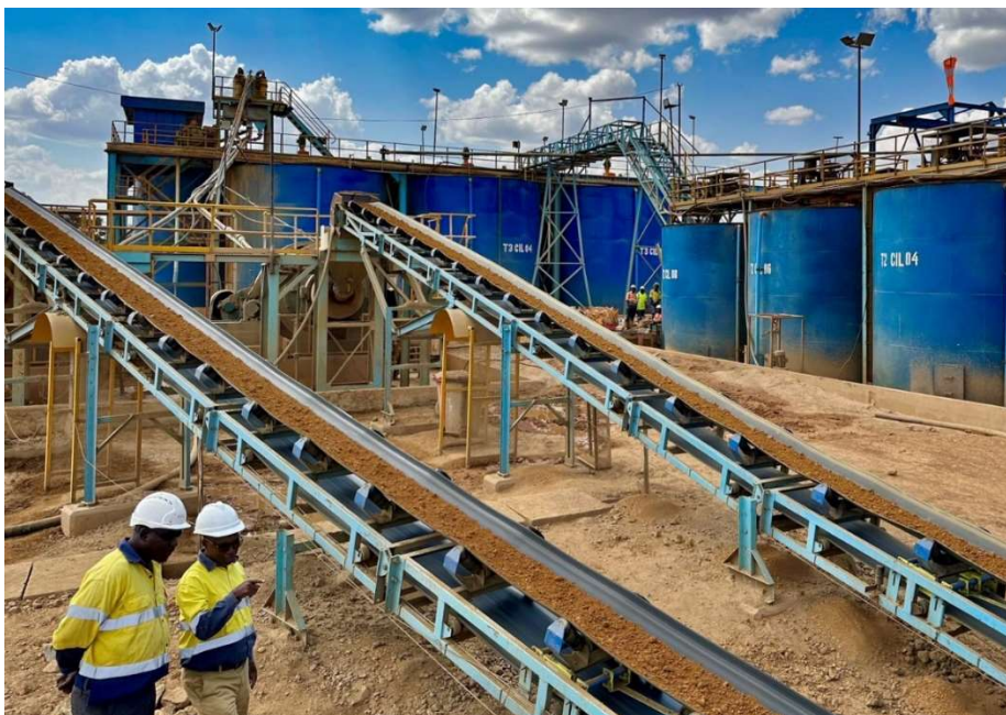
Figure 3: 1,000+ tpd Processing Plant at Buckreef Gold Mine, showing new CIL tanks and conveyor feed to the new ball mills (Q3 2023)
