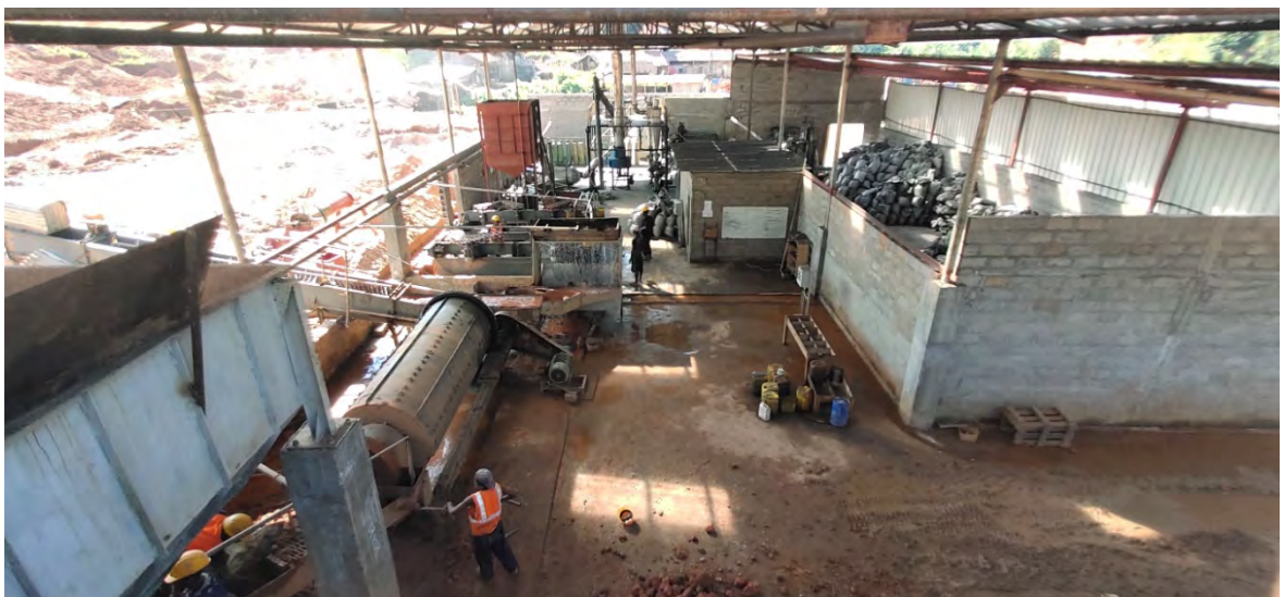
Figure 7-3: Another view of the Plant built in Sahamamy
