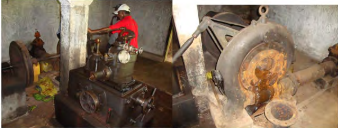
Figure 8-8: Turbine and other equipment at the old Hydro power plant (now non-operational)
