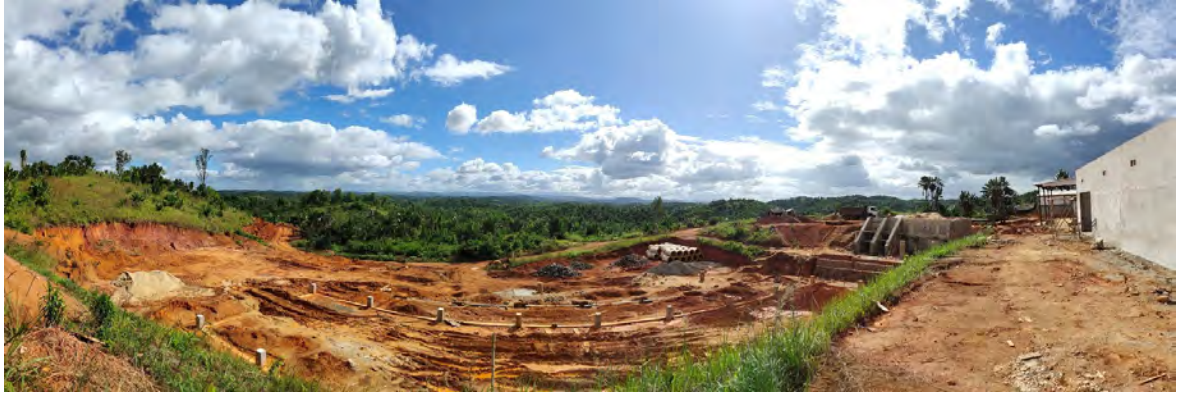
Figure 7-5: Vatomina: View of the Construction site taken during SRK site visit in 2019
