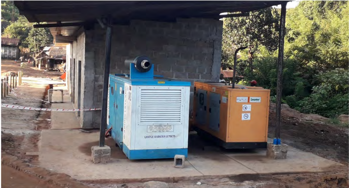
Figure 8-6: New Generator installed in Sahamamy replacing the old unit inherited with the acquisition
