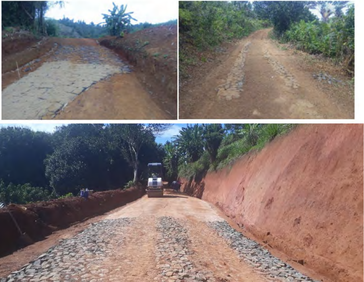
Figure 8-10: Compactor (introduced in August 2019) at work in Vatomina; to be used for road management
