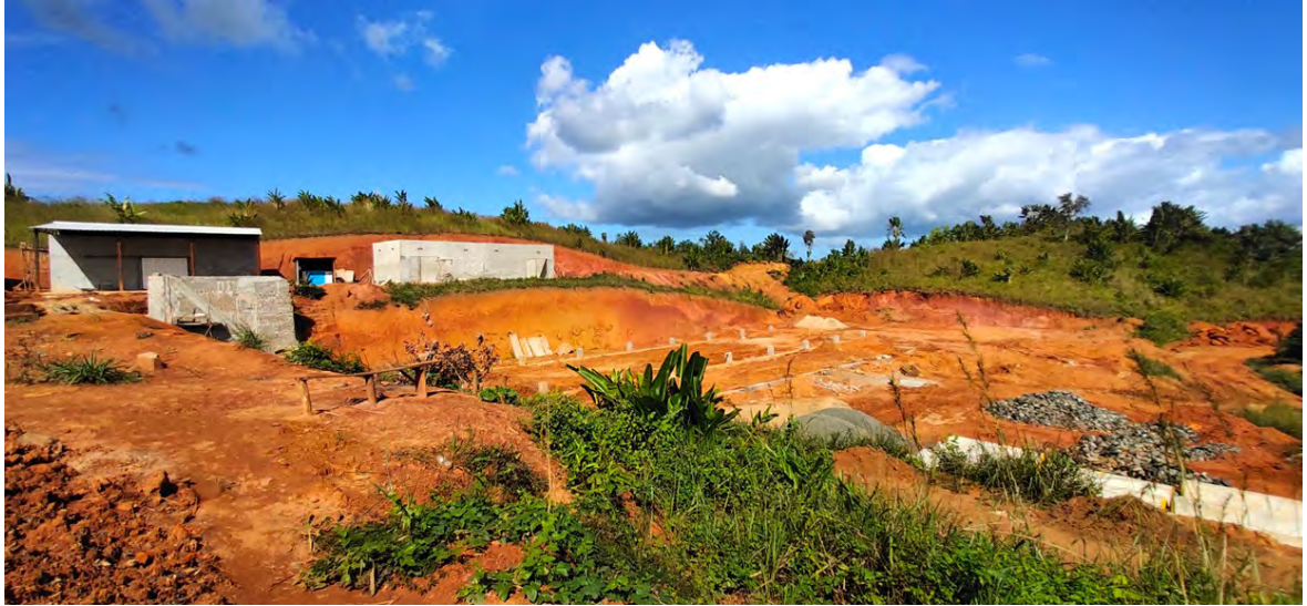
Figure 8-14: Area where the 1st Stage Processing Plant (6,000 tpa) is planned; picture taken by SRK during site visit
