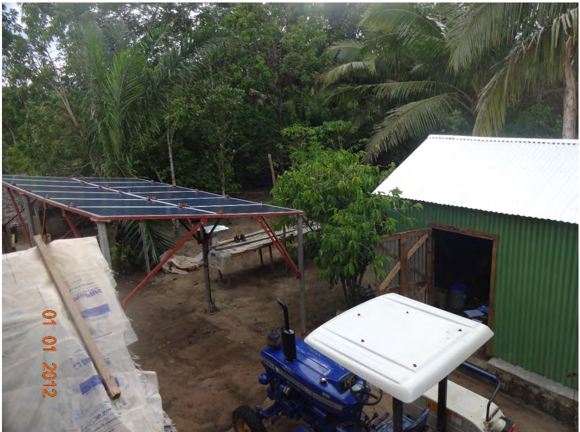
Figure 8-12: Store and a Solar power pack at the Vatomina Base Camp
