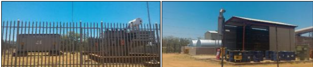
Figure 8.4.3: 22kV substation, transformer and switchgear installation (Left Hand Side) and existing main diesel generator house (RHS)
