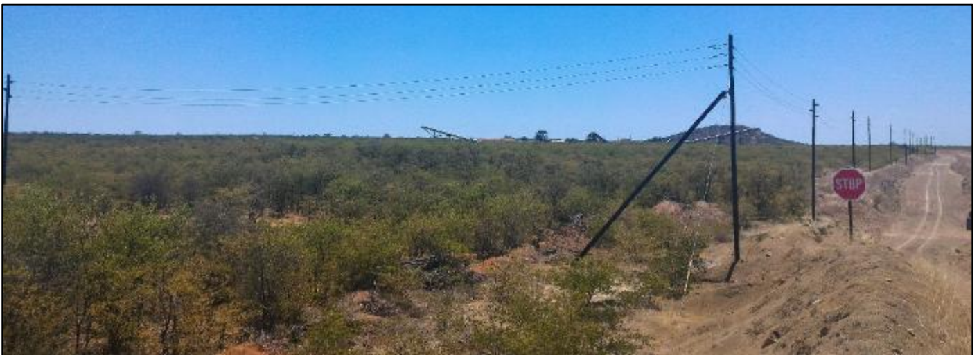
Figure 8.2.4 Power line has been extended to the contractor's yard. Existing plant in background
