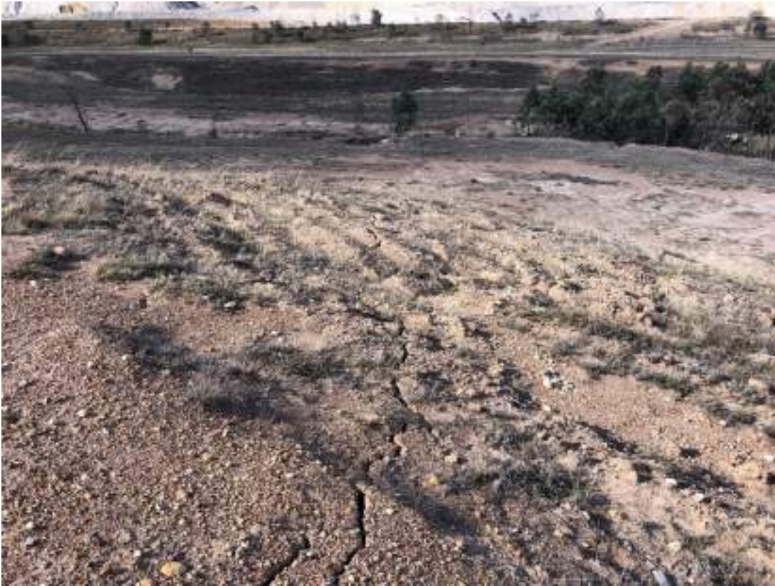
Plate 28. Subsidence cracks, erosion and bare soil along the North Wambo Creek Diversion near site 23R
