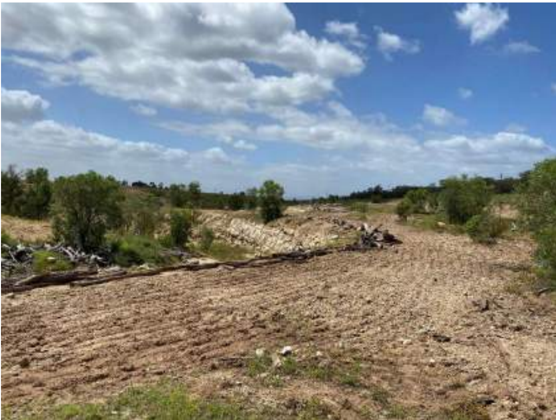
Photograph 22: Example of active soil remediation work in the North Wambo Creek Diversion area in 2020
