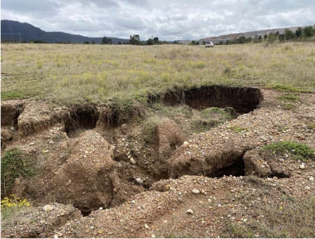
Photograph 18: Gully erosion within the North Wambo Creek Diversion (near site 23R) in 2022
