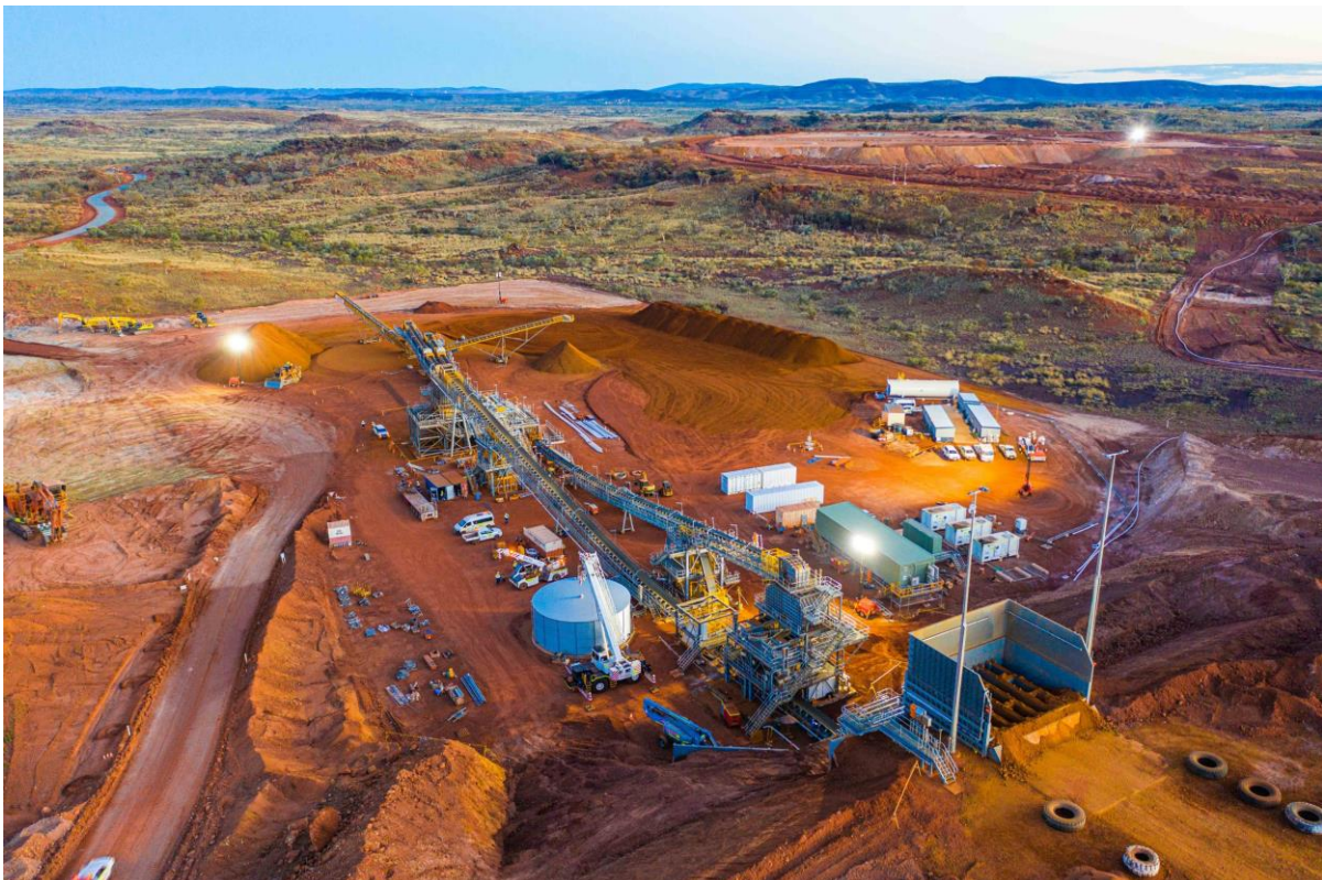
Figure 17-1 Process Plant at the Wonmunna Mine (Mineral Resources 2022)
