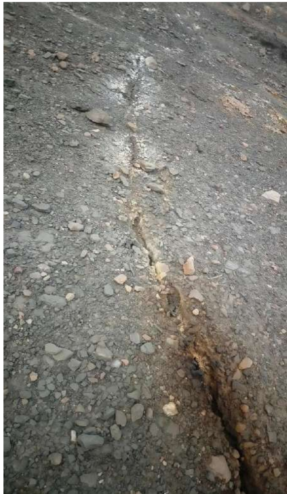
Figure 20: Fume cracks in the Bhulanbarari area.
