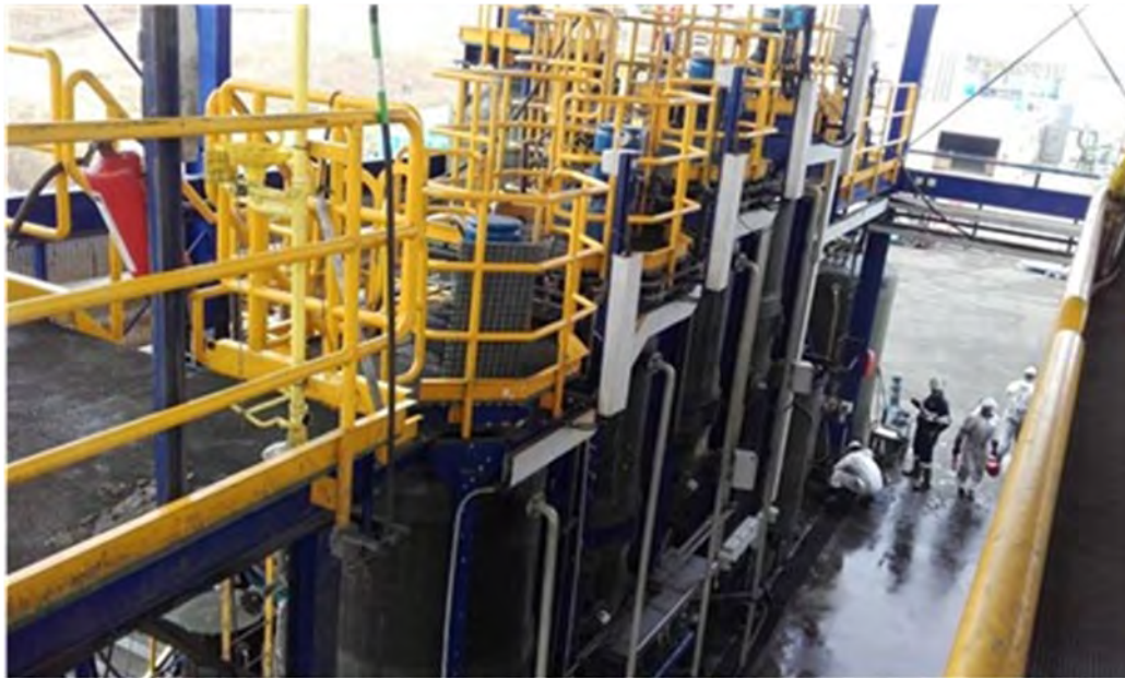
Figure 13-4 4 Pilot Plant Leaching Reactors
