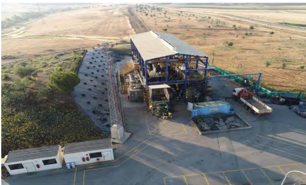
Figure 13-3 3 Pilot Plant Aerial View
