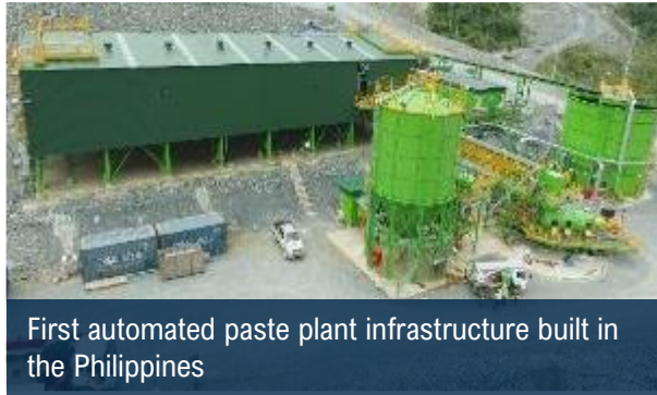
PASTE BACKFILL PLANT
