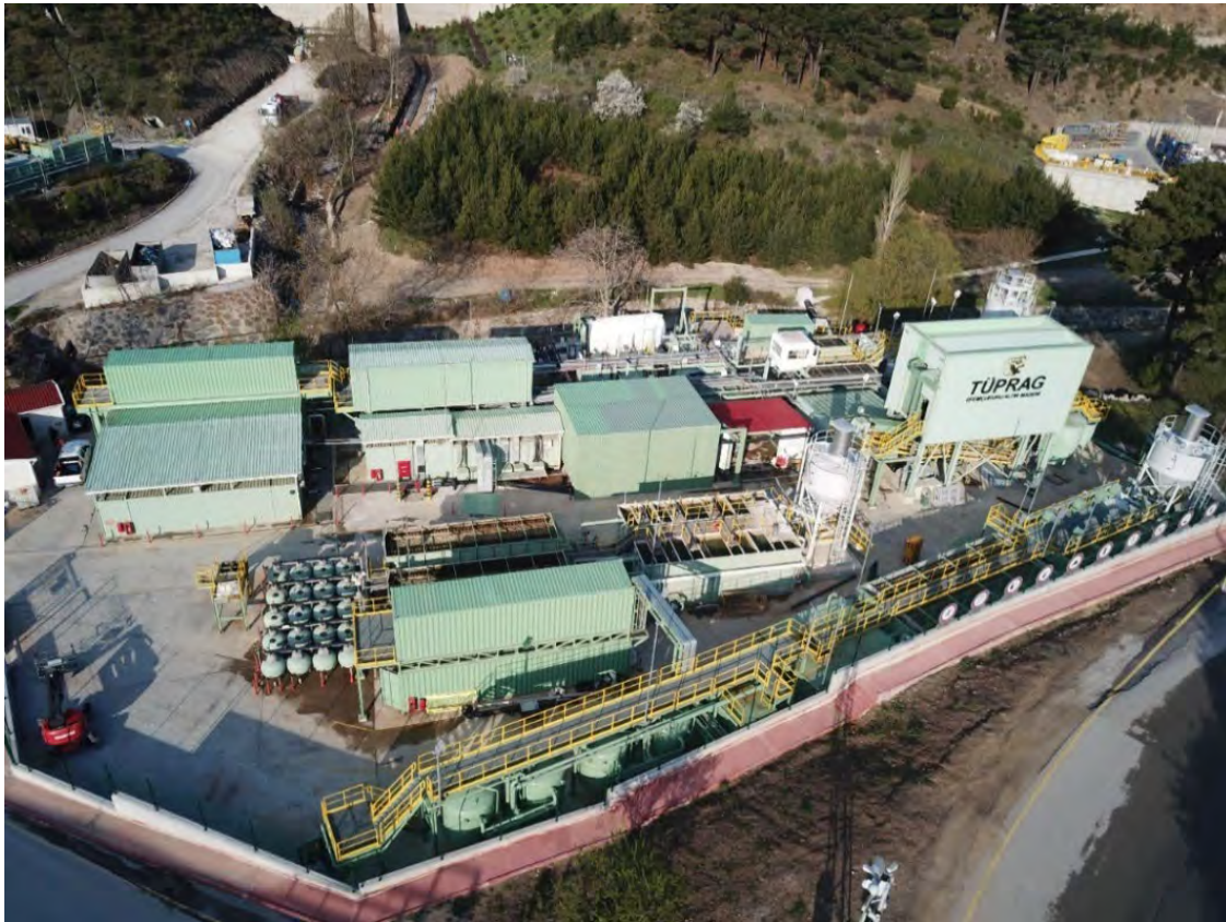
Figure 18-7: Water Treatment Plant (Eldorado, 2019)
