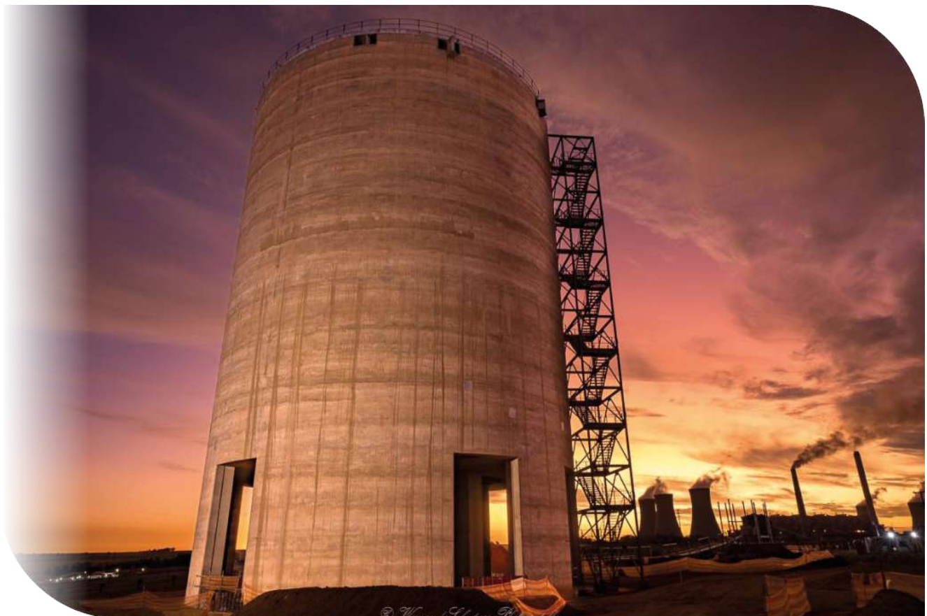
Buffer silo between Mine 1 and Matla power station
