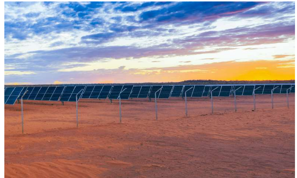
Solar panels at our Granny Smith mine in Western Australia
