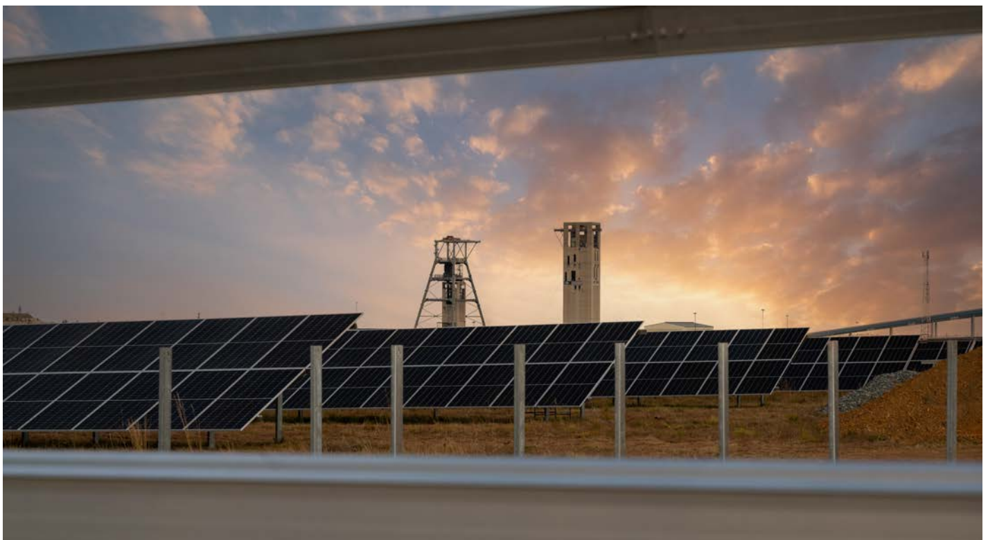
Solar facility at the South Deep gold mine
