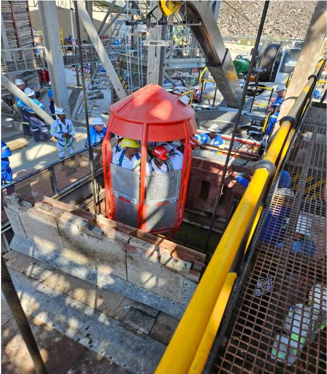
Figure 16-67: Mobile Emergency Winder Commissioning 2023
