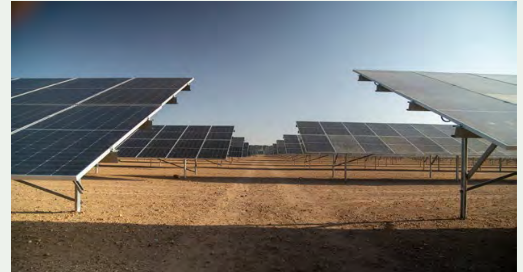
At Tasiast, a view of the solar plant.
