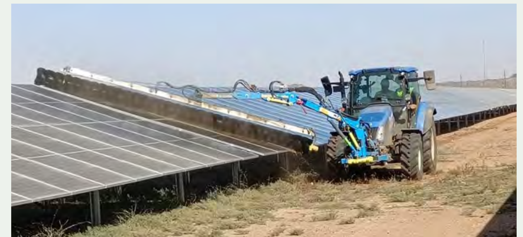
At Tasiast, we have invested in a mechanical cleaning system to manage dust levels efficiently.
