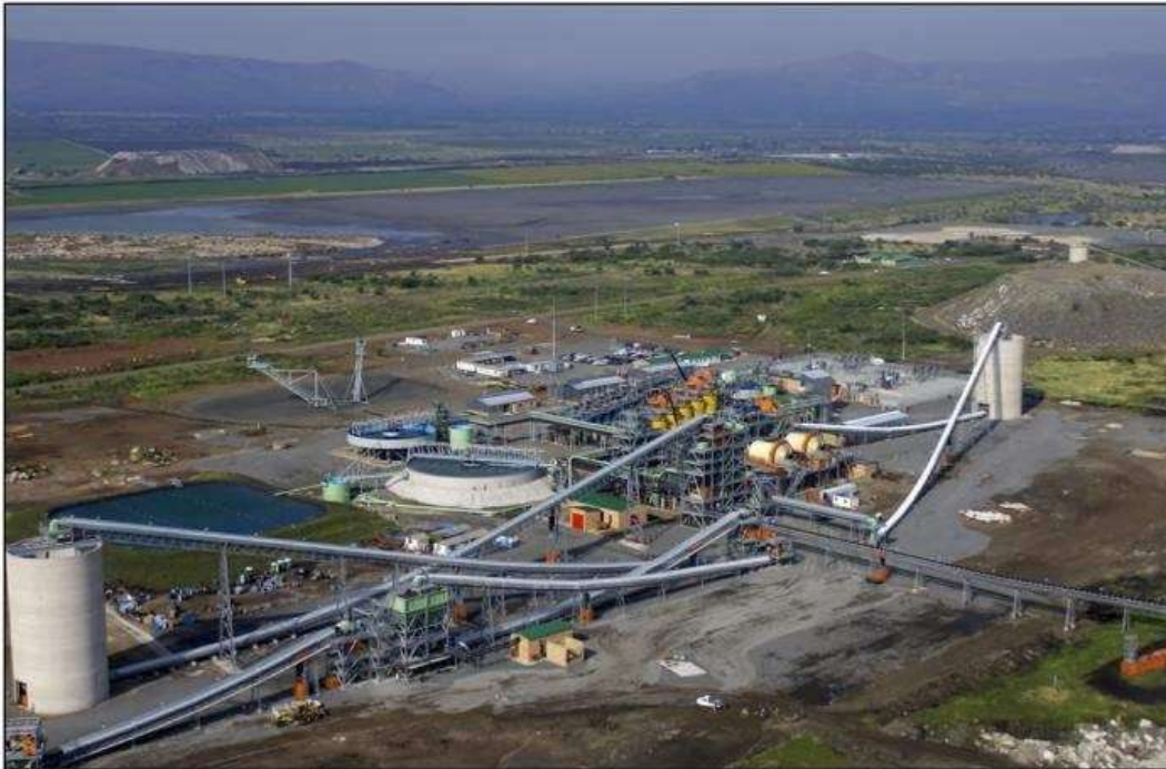
Figure 40: Aerial View of the K2 Plant
