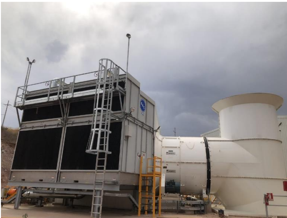
Figure 18.4: Air Intake through Cooling Fins with Cooled Air Delivered to the Underground
