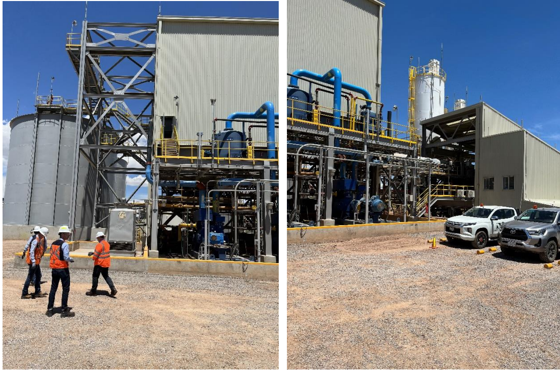
Figure 18.9: Filter Feed Tanks (left), Vacuum Pump, and Binder Silo (right) at the Paste Fill Plant
