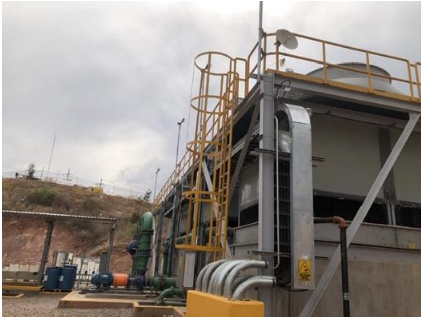
Figure 18.3: Evaporative Cooling Towers as the First Stage of Cooling
