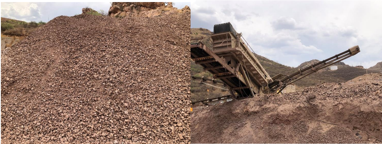
Figure 18.7: Astec KCI-JCI Mobile Jaw-cone Crushing Plant (left); -76mm Aggregate Stockpile (right)
