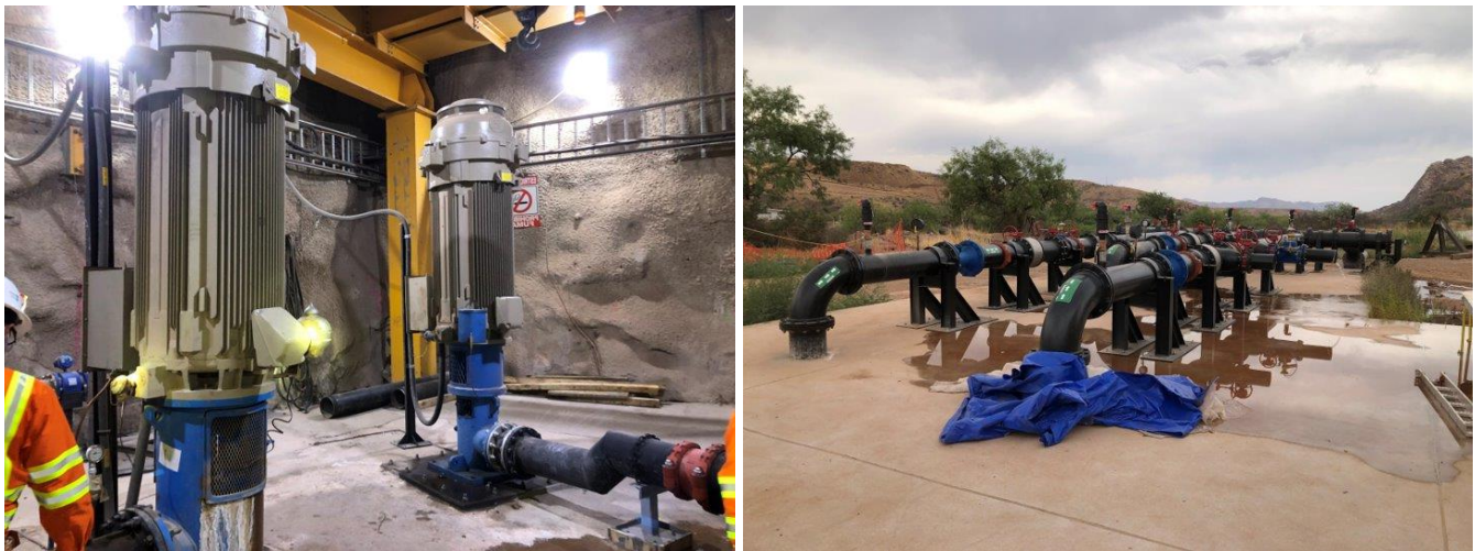
Figure 18.5: Underground Wellhead Pumps and Surface Discharge Header
