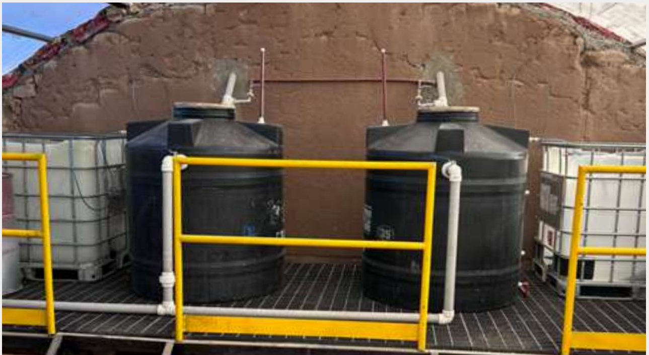
Anaerobic biodigesters for the pilot treatment of organic waste
