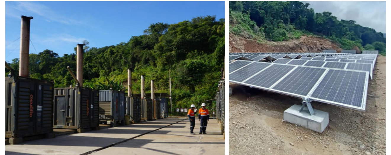
▲ Genset dan solar panel di BKP-BTR Genset and solar panel at BKP-BTR
