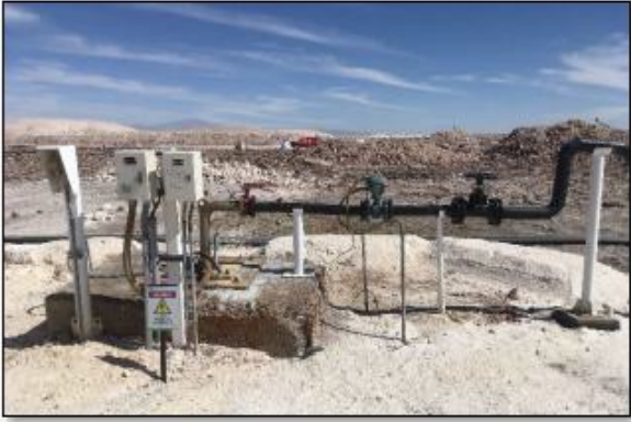
a) Brine production wells with surface equipment
