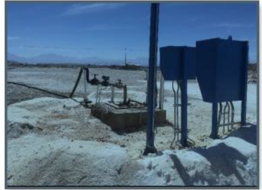
b) General view - production brine well and HDPE pipe for directing brine to the homogenization ponds
