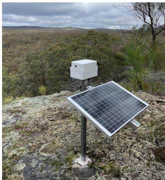
Photo 3 GNSS Unit within the BCA (August 2022)
