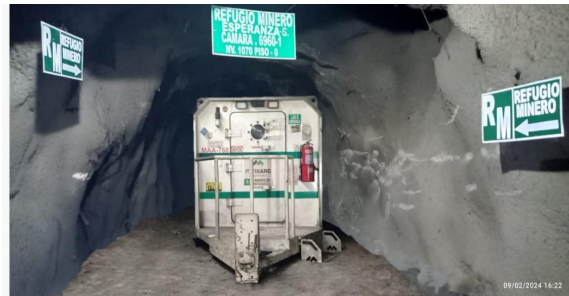
Figure 18-6: Yauricocha Esperanza Sur Refuge Chamber
